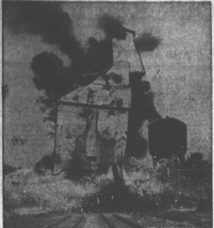
BLASTED ACCIDENT—Taking spiteful vengeance on the Rock Island Railroad, this unseamed coal chute has its supporting columns blasted away, and settles right on the main line. Engineers had set their explosive charges to throw it clear of the tracks, but the outmoded structure wouldn't cooperate.
