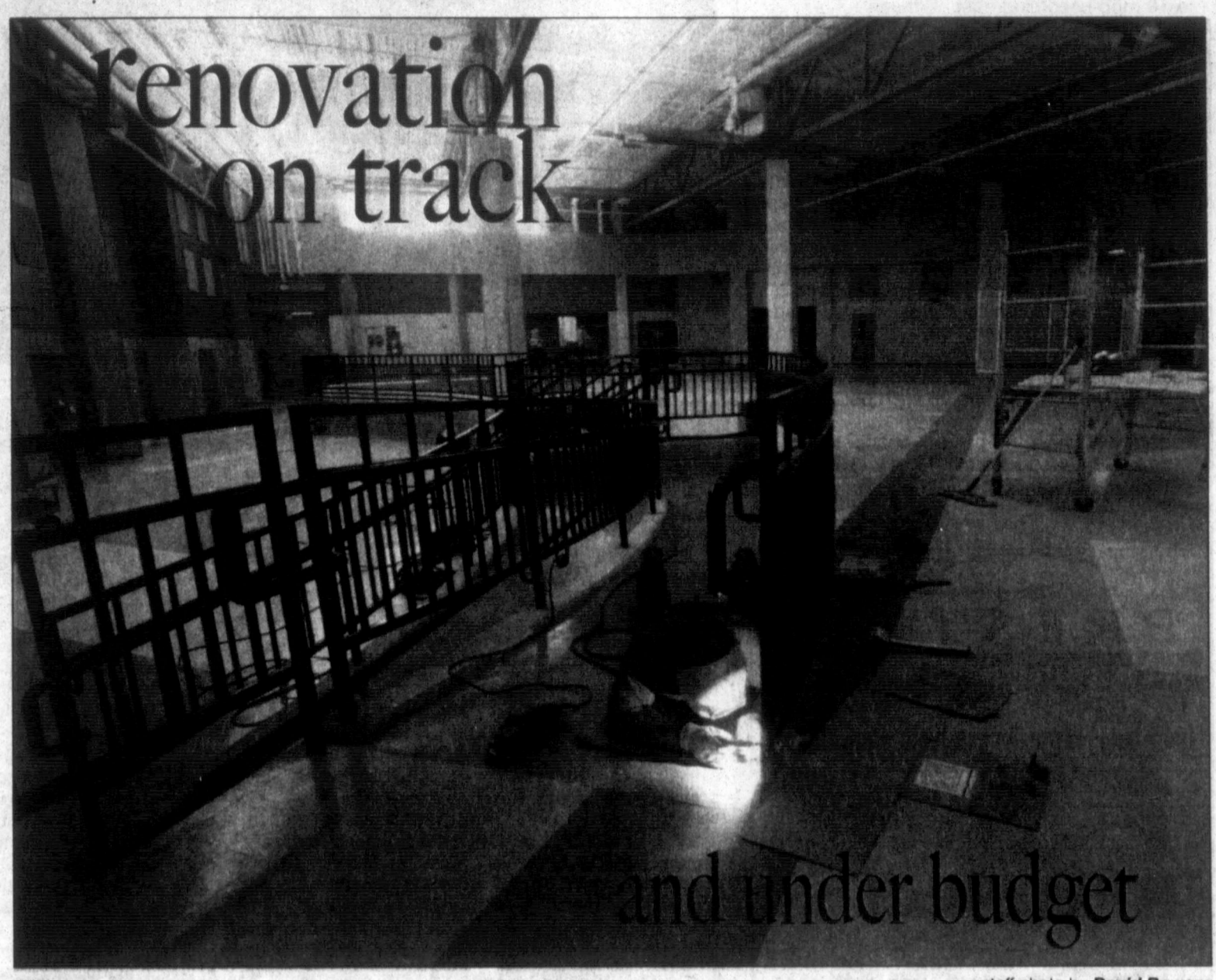
Getting the Pampa High School commons ready for opening day, Chris Urteaga welds cross pieces into place on handrails in the commons area. Jeff Popp with Western Builders said that while there will still be some work left to do, the renovated building will be ready for students and teachers when school opens in August.
