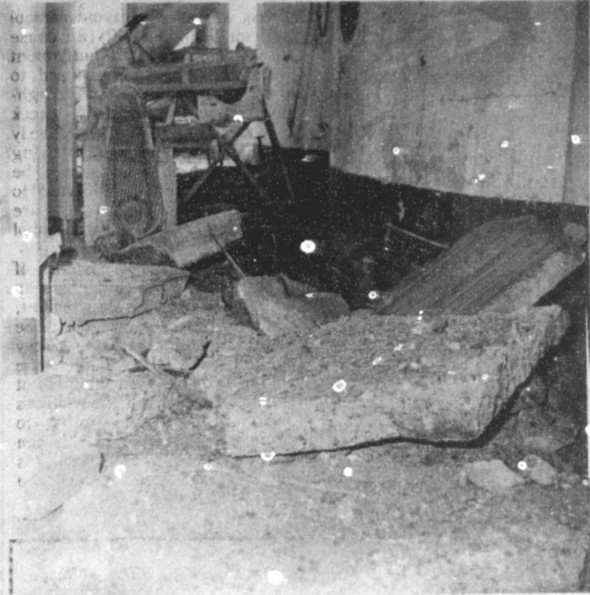
FOUNDATION EXPLODES —On the east side of the elevator at Farmer's Co-op Elevator, this is what a six-inch thick foundation looked like Tuesday afternoon following an explosion at the elevator.
