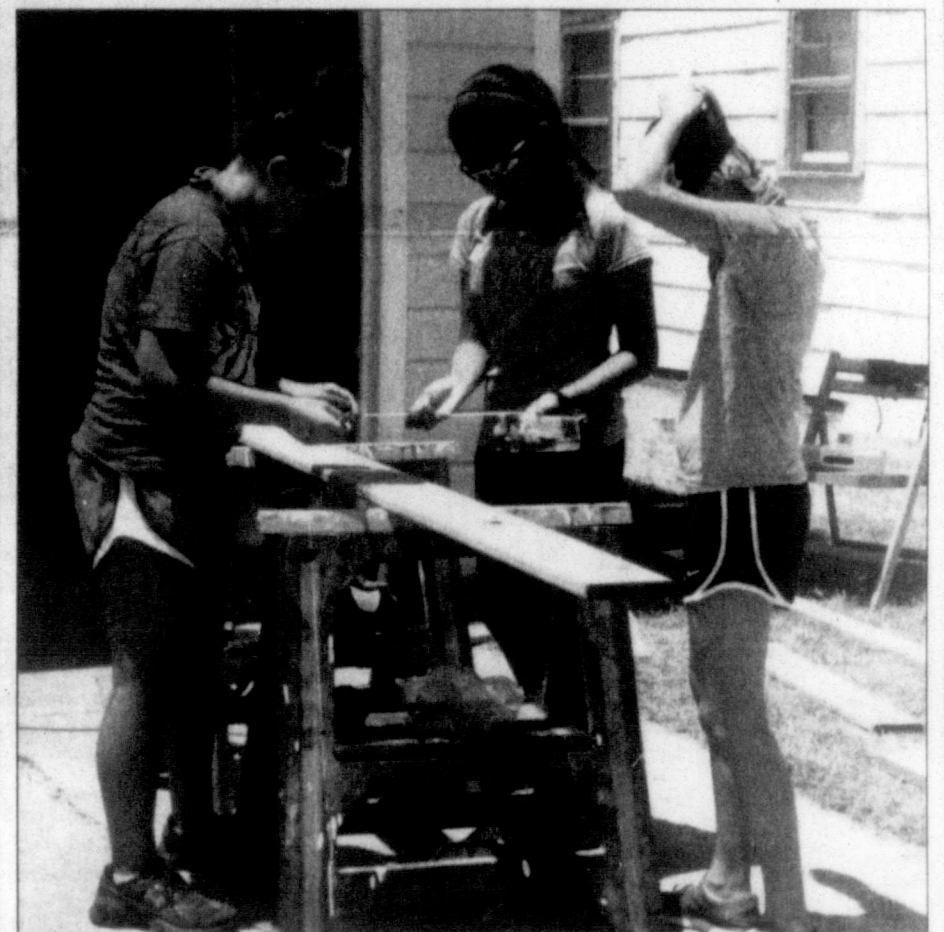
staff photo by Mollie Bryant Brittani Castillo , 13 (from left), Brienna Martinez, 15, and McKenna Hopper, 12, of Temple, prepare a two-by-four for construction of a Pampa resident's wheelchair ramp. The teens are part of a Reaching Others Through Christ, a group that performs outreach projects all over Texas.
