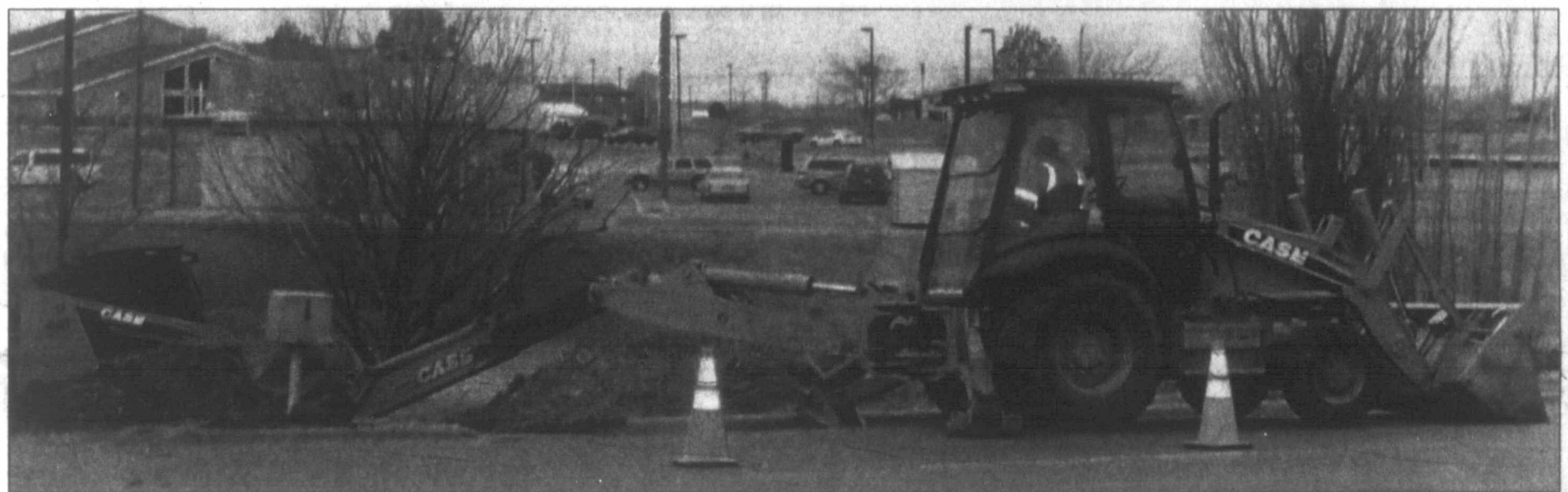
City construction crews work to install a water line near the intersection of Hobart and Somerville on Thursday.
