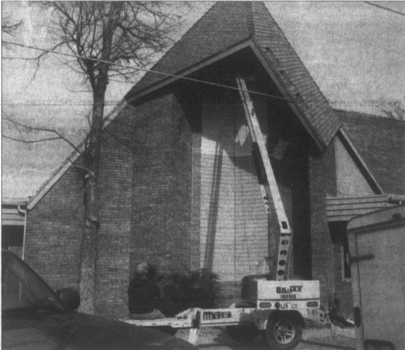
staff photo by Mollie Bryant No, that crane isn't Harvest Bible Church roof. The church's windows are undergoing repairs, with Harley Knutson (bottom left) treated to a front row seat.
