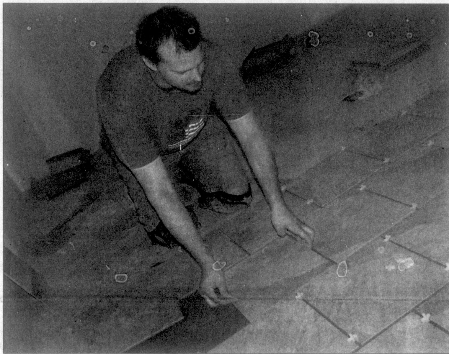
staff photo by Arnie Aurellano Daniel Lee of The Floor Store lays down square tiles to complete a floor at the soon-to-be Enbridge office in the north-west corner of the Coronado Center on Wednesday afternoon.
