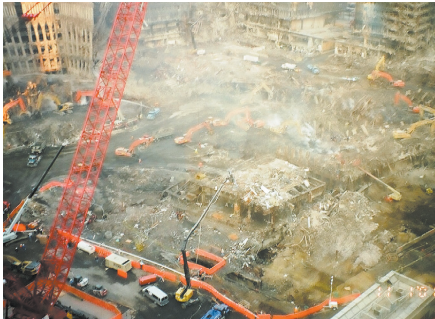
I took this shot from about the 20th floor of the World Finance Center Building II sometime around mid October. Rising 400 feet above Ground Zero stands Big Red, the largest mobile crane in the U.S.A. It was perched on the spot that was once the World Trade Center 1. The Houston company that owns Big Red flew the American flag at its peak, just above the flag of Texas. Grapplers the size of semi trailers worked 24/7 in the dust and haze that never goes away. In the background on the left, the skeleton that was World Trade Center 2 leans against the remains of buildings 8 and 9. '
