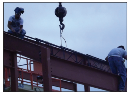
Photo by Timothy P. Howsare Construction workers were erecting a steel frame Wednesday for the new Pampa Animal Shelter, which is expected to open in the late fall.
