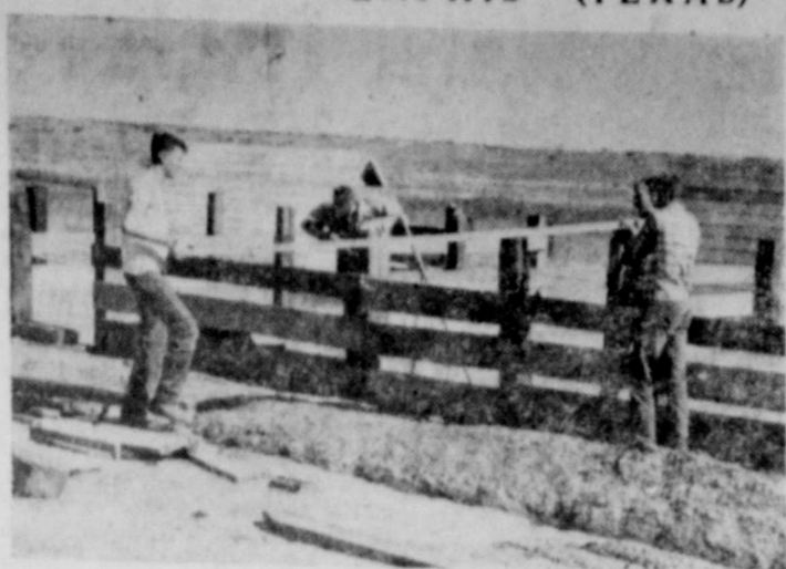
PENS FOR PORKERS —FFA boys at Boys' Ranch build new hog pens and hope in the near future to be able to raise the majority of their own pork at the Ranch. This is the first time the Ranch has had an FFA Chapter and the boys are really working to make it one of the best in the area.
