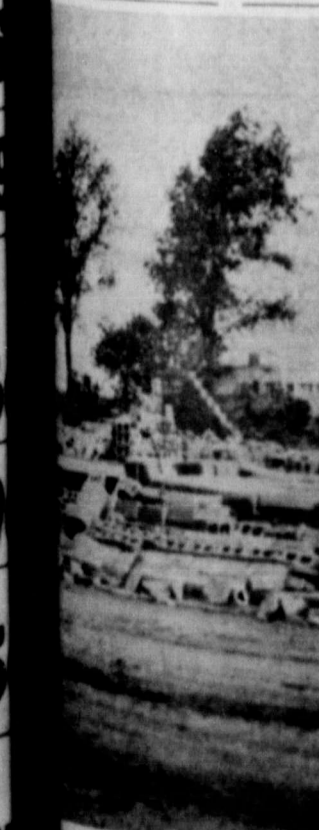
PHONE BUILDING —High winds Friday blew down four walls of the General Telephone Co. division office under construction here. The walls were 90 per cent complete before the storm hit and were completely leveled. Delay due to the mishap will be about three weeks.
