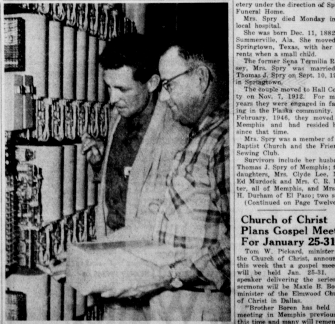
INSPECTING LINE FINDERS —Pictured above are R. R. Cole (left) and C. E. Maddox examining line finders, which are the first piece of equipment activated when a subscriber starts to make a call. Area residents will be able to see these and several other interesting pieces of equipment at the General Telephone Company's open house tomorrow (Friday) afternoon.
