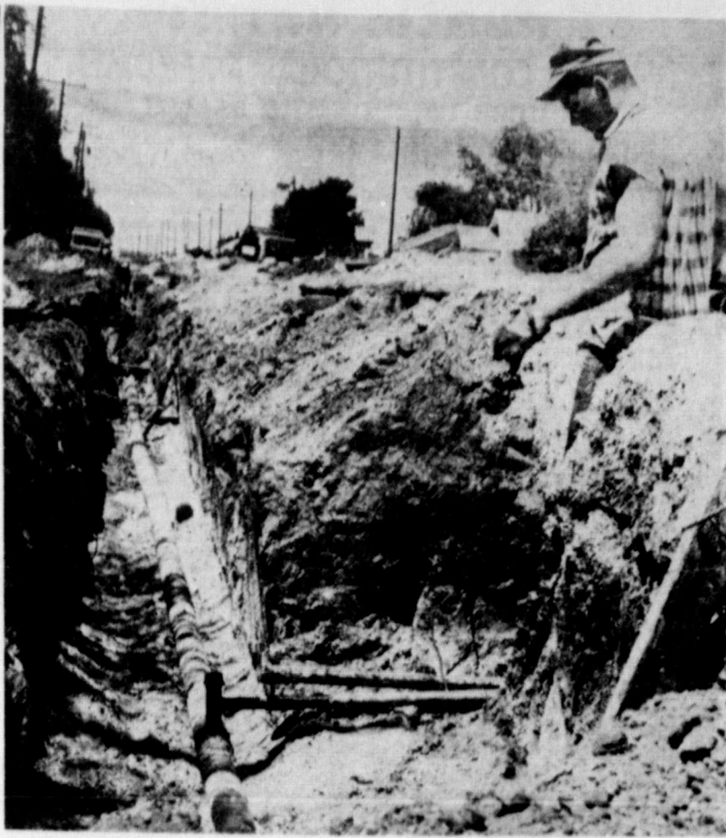
GETTING READY FOR WINTER—For the past several weeks Lone Star Gas Co. has been working in Memphis replacing old line. The picture above was taken on 12th Street recently where about two blocks of line was being replaced.
