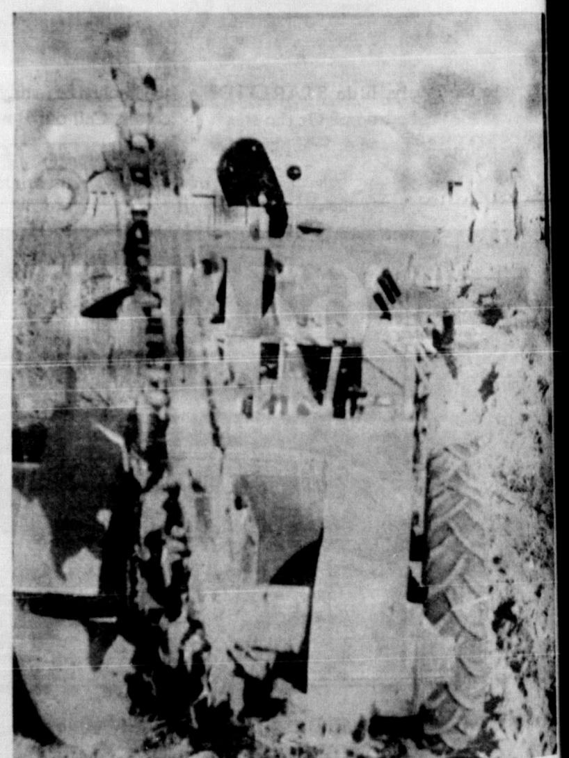
Laying underground cables for General Telephone Co. to serve residents of this area
