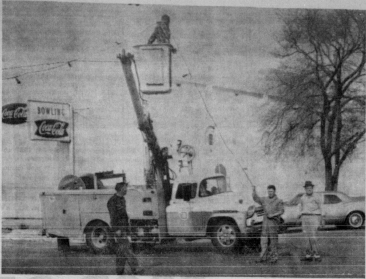
CHRISTMAS LIGHTS —Crews from West Texas Utilities and General Telephone Co. of the Southwest are shown erecting Christmas light strings around the square Monday. These lights will be turned on for the first time Thanksgiving evening. Driving the GTC "bucket" truck is Dwaine Floyd of Memphis and in the bucket is Bill Cummings of Memphis, both local employees of the telephone company. On the ground handling the lines are James Jeffers, Judge Chappell and E. M. Murphy, all employees of West Texas Utilities Company, here. The Chamber of Commerce is having a homes and business window decorations contest this year so Memphis should be well decorated for the Christmas Season.
