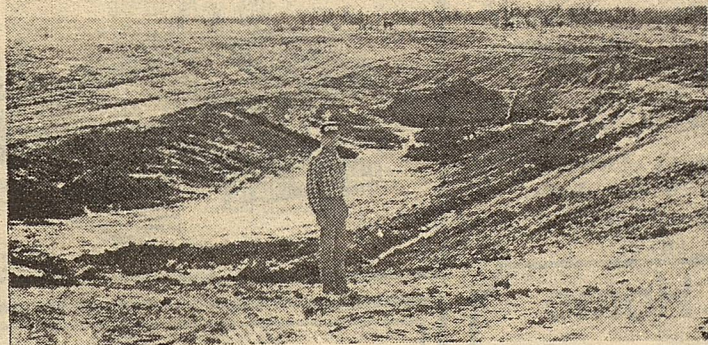
The Soil Conservation Service assists farmers and ranchers in planning and constructing ponds for erosion control, stock water, and recreation. The pond site shown here is on the Max von Roeder farm northwest of Snyder.
