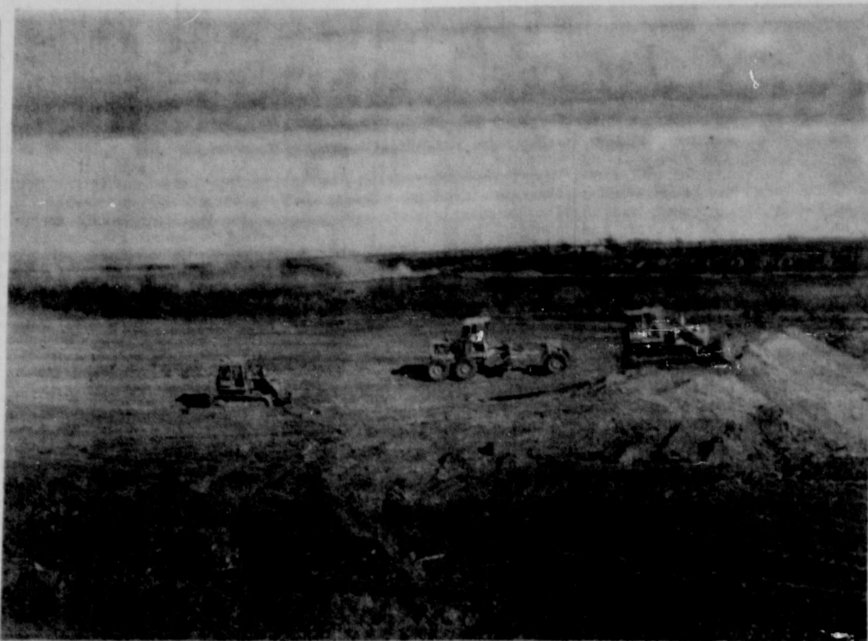
SEWAGE POND —Pictured above, City of Memphis crew is shown digging the bottom of a sewage water storage pond at the Memphis Sewage Plant located in southeast Memphis. Work began Monday on the pond which will hold over-flow water from Pond No. 2 of the system and prevent any water from the plant from going into the creek.
