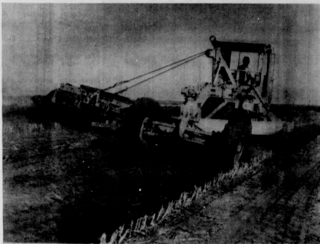
One of two elevating graders owned by Childress Dozer Service moves soil about 23 feet from the cut to the top of a terrace. This results in a high and wide terrace.
