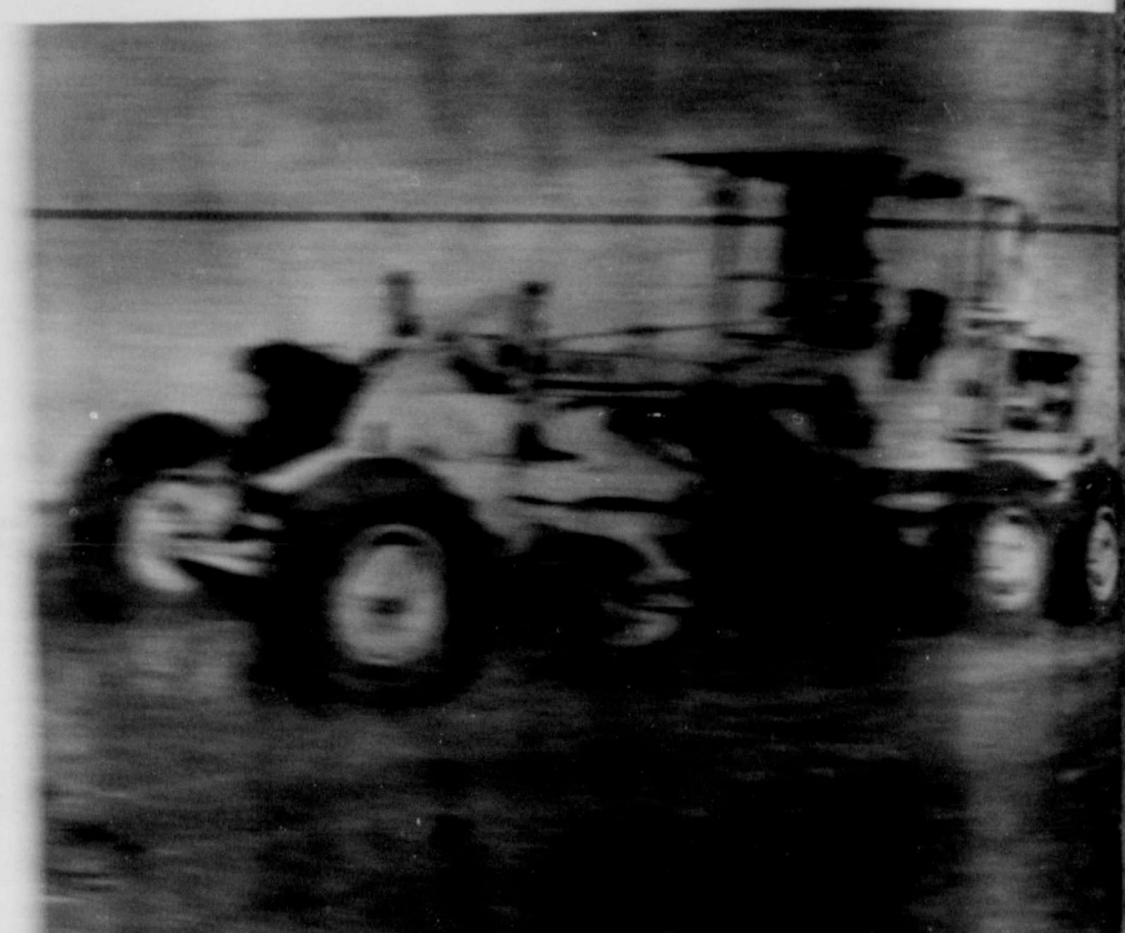
One of two motor graders is used to finish off the terrace. Two dozers are used to fill in breaks and construct cut banks. The use of two dozers, two elevating graders and two motor graders permit Childress Dozer Service to relevel approximately six miles of terrace per day.
