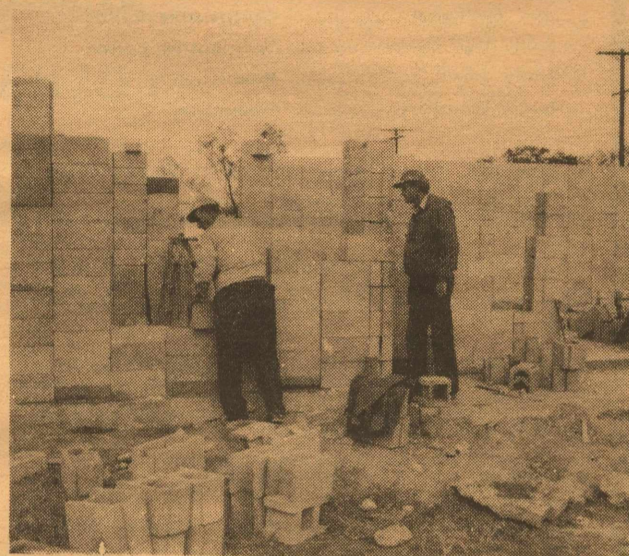
Work continues on the new home of the Kinney County Land Company.
