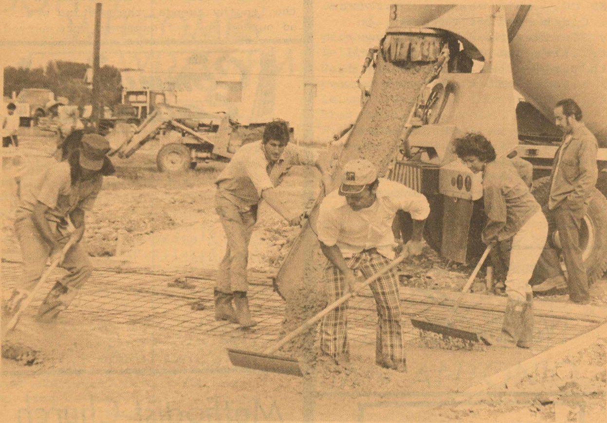
A week ago Baker Construction Company was in the process of pouring concrete for the LONGHORN RESTAURANT, 3 miles west of Brackettville. Today, if you drive by this site, the building frame is already erected----- Another Sign Of Our Progress.
