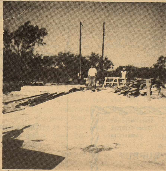
There was a house being built here on Fort Clark Springs across the road from Camper's World.
