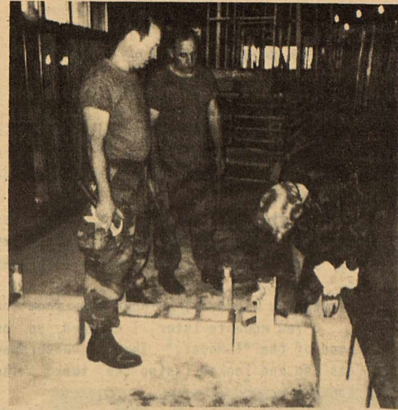
TSG. T. Oakley, SSG. F. Misko, and TSG. D. Price work on the interior walls of the new building.
