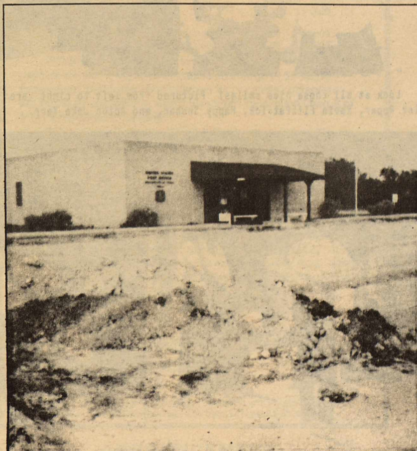
Pictured above is the U.S. Post Office located in Brackettville. It is in the process of getting a new cement parking lot.
