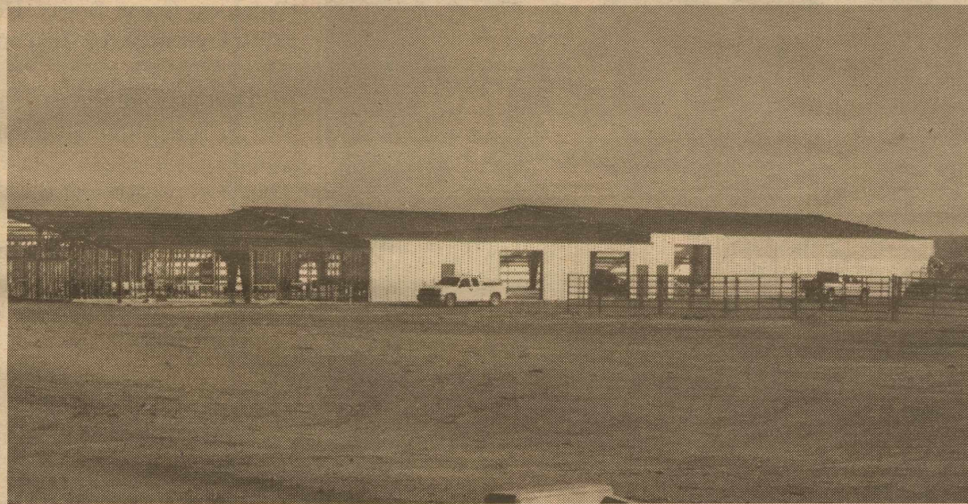
Construction on the brand new Borden County Event Center is well on it's way. Borden County Judge, Van York, says completion of the Arena and Event Center is scheduled for January 2011.
