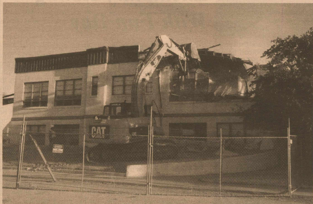
Construction crews began demolishing the old Borden County 2-story school building last week to make room for construction of the new softball field.
