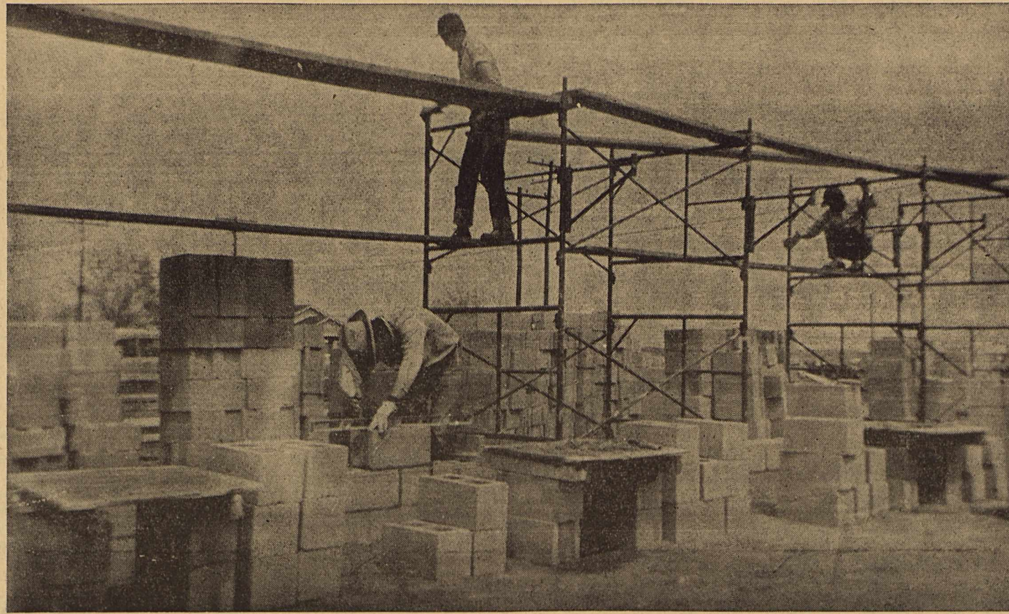
THE PHOTO above is of the building Joe Curry is constructing. Work on it had to be started all over this week after high winds blew it down Saturday.
