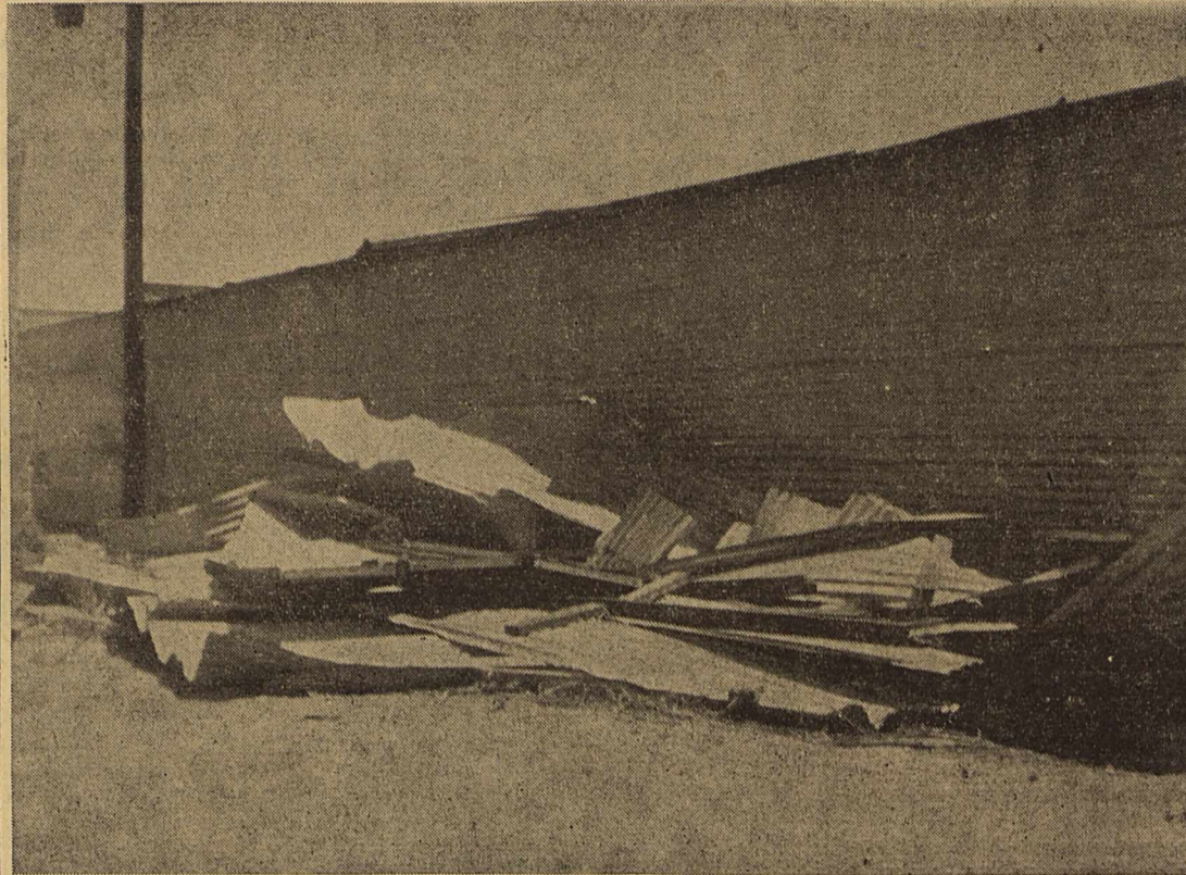
HIGH WINDS which hit Plains Sunday after noon literally blew the roof off the sheds at the lumber yard. Little damage otherwise was reported by local residents.
