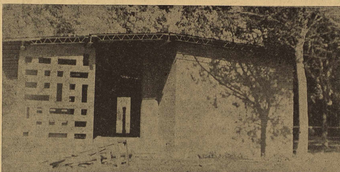
EXTERIOR WORK ON THE YOAKUM COUNTY LIBRARY here is nearing completion. The roof is nearly finished, and plastering is to get underway Monday morning. Brick work on the structure is almost done, according to workmen on the project. REVIEW PHOTO
