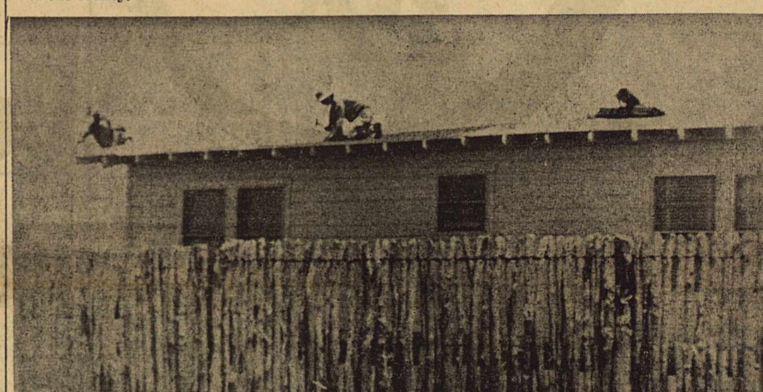
WORKMEN WERE BUSY on the D. C. Newsom home this week, repairing the damage to the roof caused by the terrific wind which hit here Monday evening. Damage to the home was estimated at $1,000.
