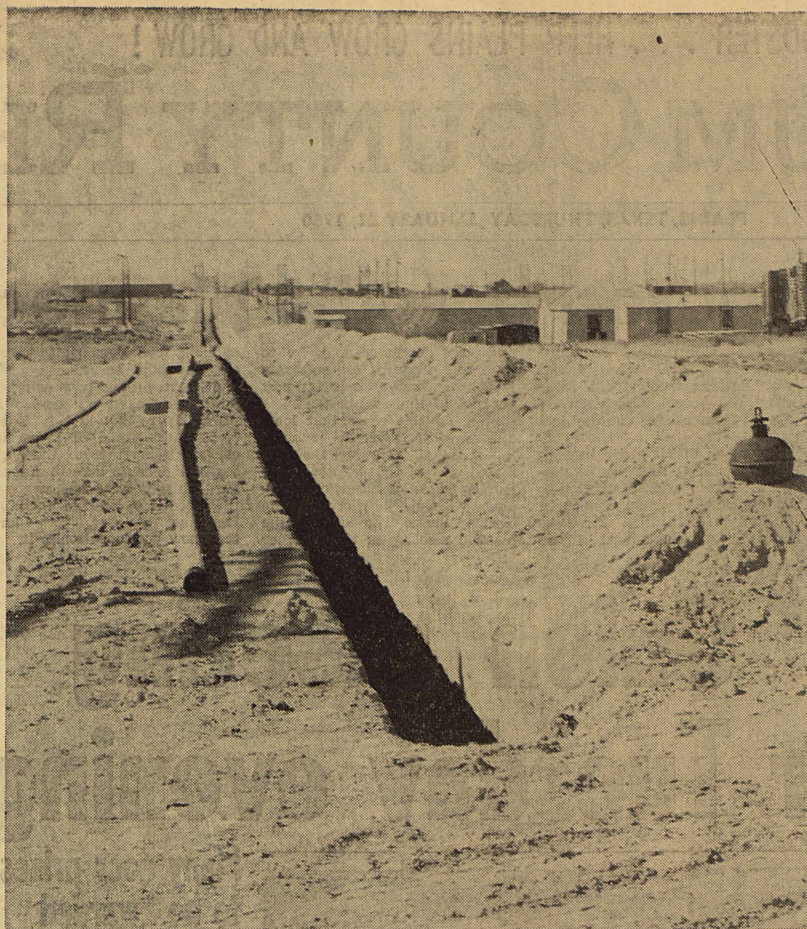
RAPIDLY NEARING completion is the new gas line being installed by the city of Plains. This picture shows a ditch which is being dug on a street in the north part of the city.
