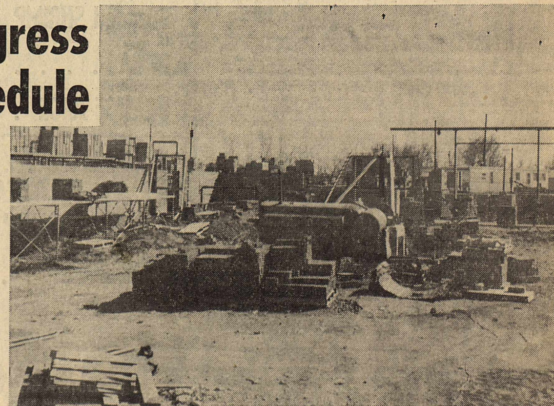
THE STRUCTURE SHOWN HERE will be the new auditorium when finished. The picture was taken from the stage which faces south. Behind
