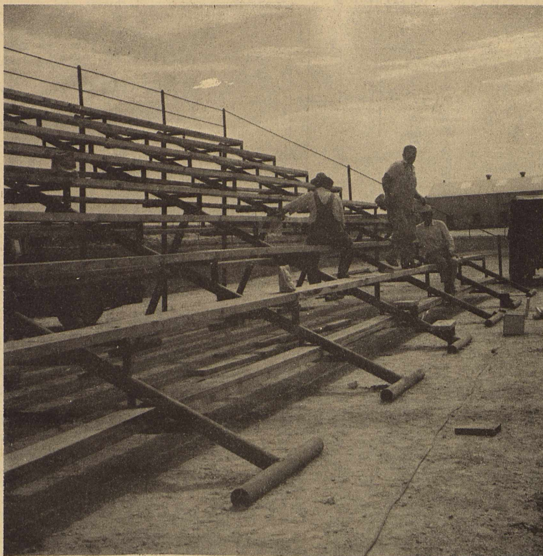
FINISHING TOUCHES--- New bleachers are being provided for rodeo spectators this year and are about ready to be put to use as workmen for Yoakum County put on the last of the lumber.
