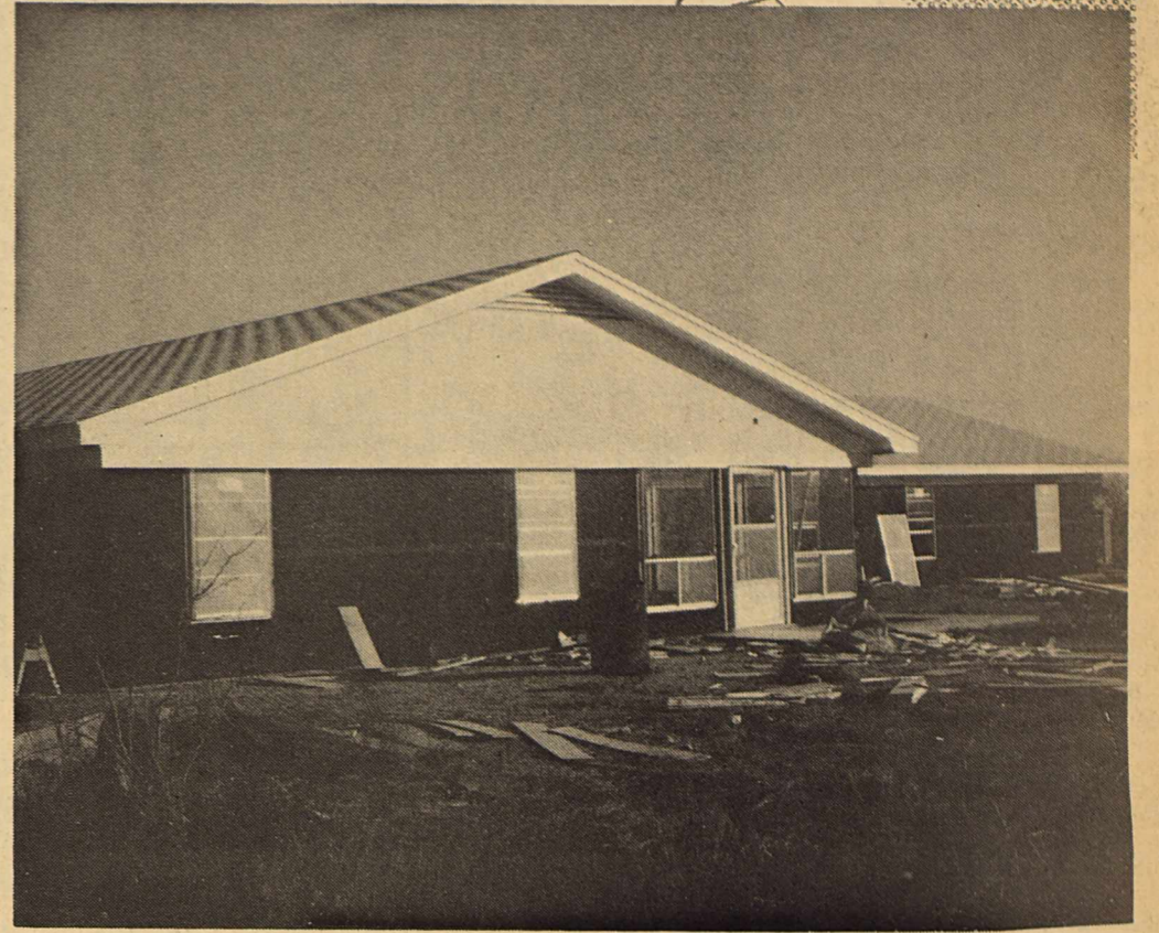
SOON TO BE COMPLETED---Is the status of the new Convalescent Home presently being built in Plains. It is a 30-bed brick structure.
