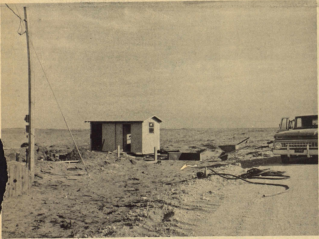
ABOVE IS A PORTION OF THE CONSTRUCTION SITE at the Yoakum County Park. This is the portion at the place where looking right, just past the entrance to the park, you would enter the playground part of the park, and just to the right of that is the actual entrance to the golf course itself.
