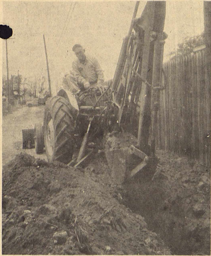
SMITTY USES NEW BACKHOE TO DIG DITCH IN BACK OF ALMA'S CAFE FOR THE NEW WATER PIPES.
