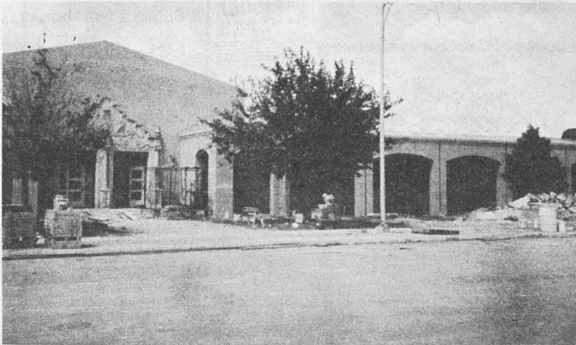
AS WORK CONTINUES on the Junior High Building, its students will be asked to enter through the back doors when school begins Sept. 3
