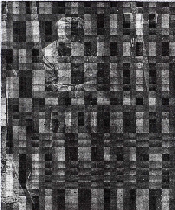
Pitching in to help on the enlisted men's swimming pool digging detail, Col. William W. Jones, the Station Commandant, operates the shovel.
