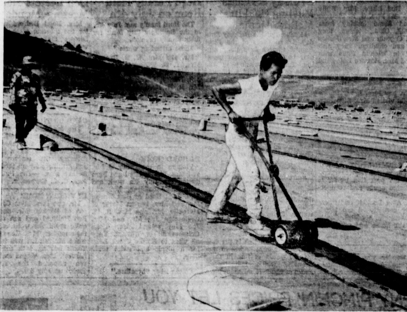
ROLLING AND SEALING a seam lap is final operation on rubber lining for Hawaii's Kualapuu Reservoir, largest rain-harvesting reservoir of its kind in the world. Its purpose is to divert misguided rainfall in Molokai which falls mainly on the wrong side of the mountains, seldom on the plains where it's needed.
