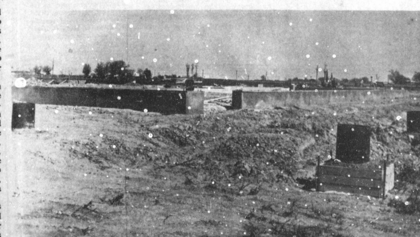
DENT FARM SUPPLY FOUNDATION --Taking advantage of beautiful spring weather, the foundation for the new Dent Farm Supply at the west edge of Muleshoe is underway. Friday morning, workmen were getting ready for the construction of the new facility. Dent Farm Supply is owned and operated by Ronnie and Leon "Tuffy" Dent, former residents of Earth and Springlake.
