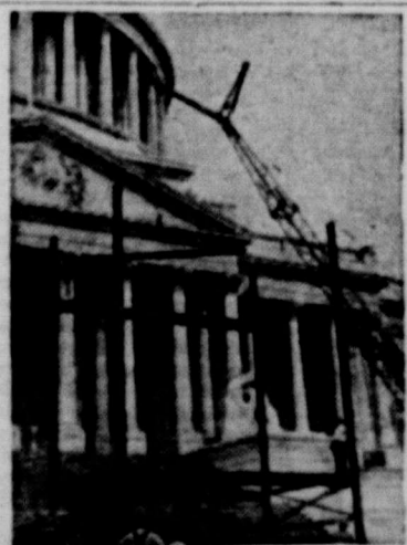
PREPARE CAPITOL . . . Steel framework for the inaugural stands at the Capitol is hoisted into place as preparations for the inauguration ceremony next January get under way. The Capitol dome also is getting a new coat of paint.
