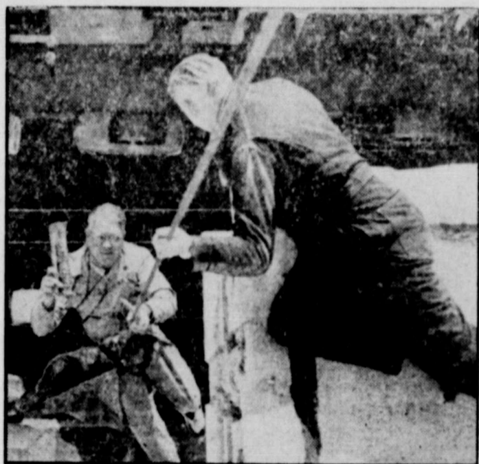
PREVENTING A HEADACHE —Steeplejack Ralph Clark, his dangerous task completed, is hoisted back to the roof of a San Francisco hotel. Clark was suspended by rope 13 stories above the street to remove a loose chunk of concrete before it could fall and cause damage. Looking down from the hotel's roof is Clark's friend.
