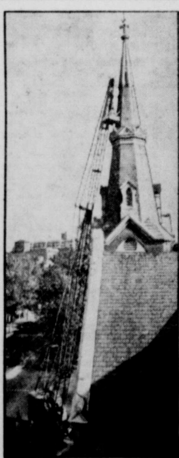
SHINGLE SHIFTER —All up in the air over his work is Jackson Davis, of Arlington, Va. Above, he repairs loose shingles on the steeple of a Washington, D.C. church. Davis, an employe of a roofing and sheetmetal company, is suspended in a wooden basket seat from a huge crane.
