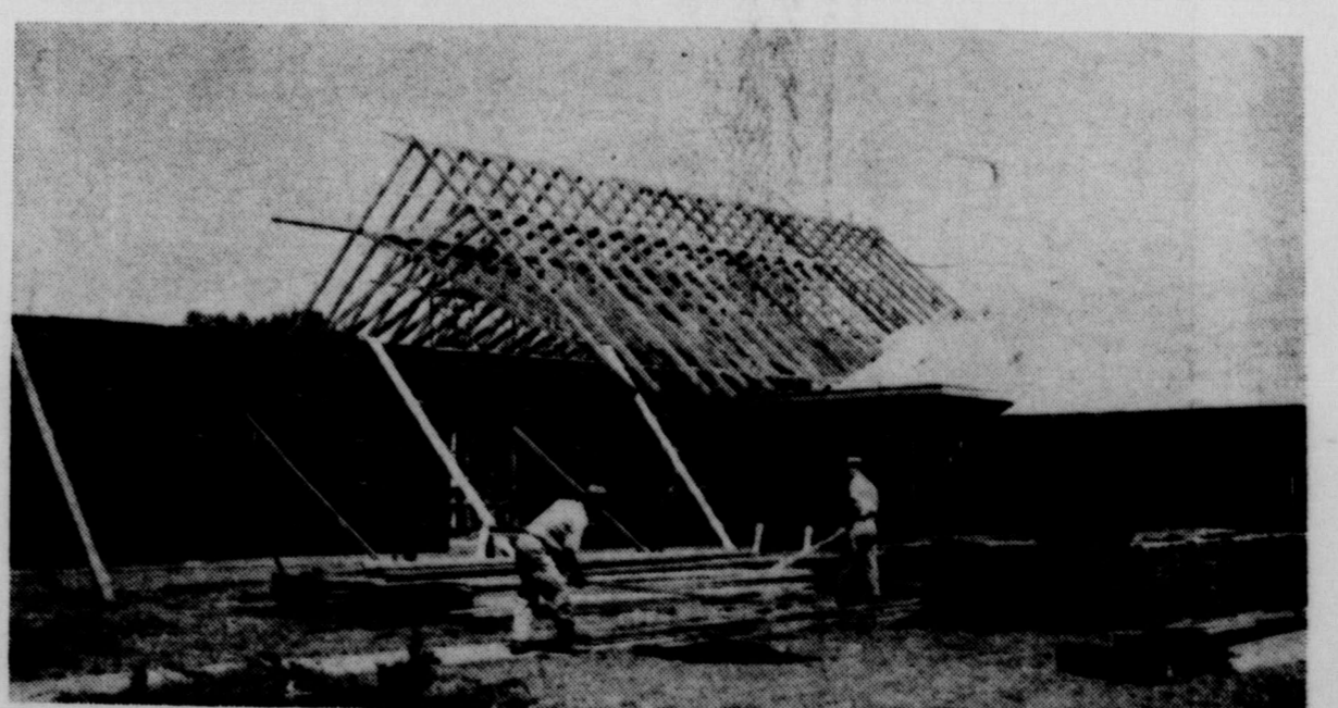
ROOFLINE TAKING SHAPE—The roof line for the new building of the First Christian Church is beginning to take shape, as this picture made Friday afternoon shows. The sanctuary will be on the left and Sunday school classrooms in the section on the right. (News photo)
