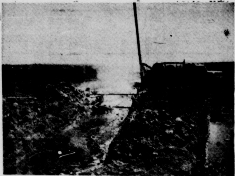
GAMBLE WELL GOES WILD —Pictured above in the cloudy portion of the center of the picture is oil and gas blowing out of the No. 1 Lucy Gamble oil well northwest of Thalia. Workmen were removing the casing to repair a gas leak last Friday morning when the well got out of hand. A high north wind carried the black gold over a large area of wheat before it was finally brought under control.
