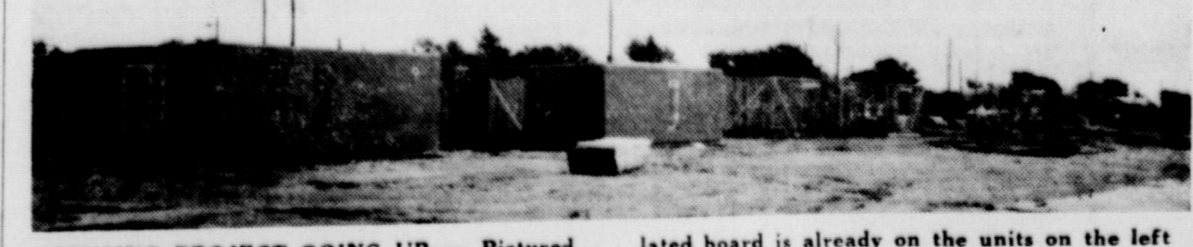
HOUSING PROJECT GOING UP —Pictured above is a scene at the new housing project under construction east of the square. Insulated board is already on the units on the left while framework is visible on the unit pictured to the right.
