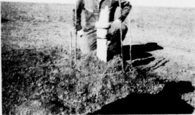
Underground pipeline installed to irrigate with effluent from pollution abatement holding pond.
