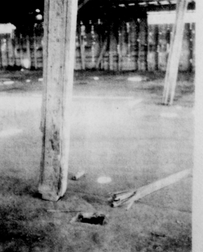
10" X 10" BEAMS DISPLACED at the Tahoka Compress when the roof was raised off the warehouse building by a force believed to be a tornado. 48 such beams were moved from their concrete resting places.
