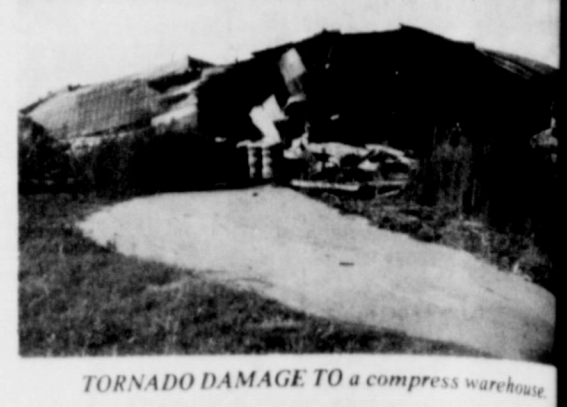
TORNADO DAMAGE TO a compress warehouse.
