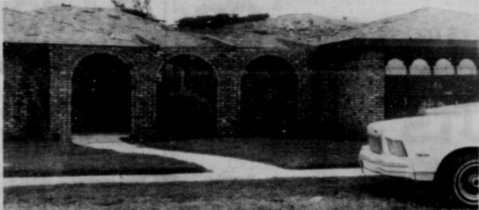
FIRE DAMAGES HOME—Fire caused by lightning heavily damaged his brick home of Mr. and Mrs. Mike Orr southeast of Tahoka Saturday night. The Orrs lost much of the contents of the home because of smoke and water damage. (Lynn County News Photo)
