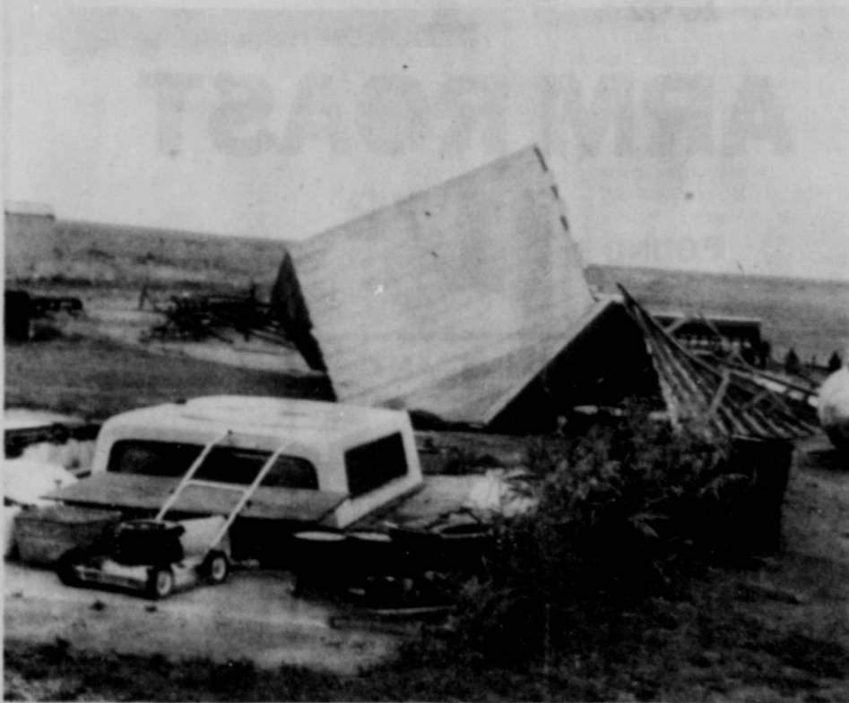
FLIPPED LID—This metal shed at the Boyd Barnes home in Draw was flipped backwards off the concrete floor by a storm Saturday night. The camper-top and other items in the shed were not disturbed. (Lynn County News Photo)
