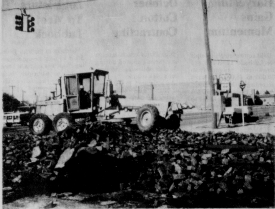
BRICK TRICKS --Texas Highway Dept. crews ripped up the bricks in the intersection of Main and U.S. 380 Monday, clearing the way for new paving of the intersection. Traffic was blocked off the intersection for most of the day. (LYNN COUNTY NEWS PHOTO)
